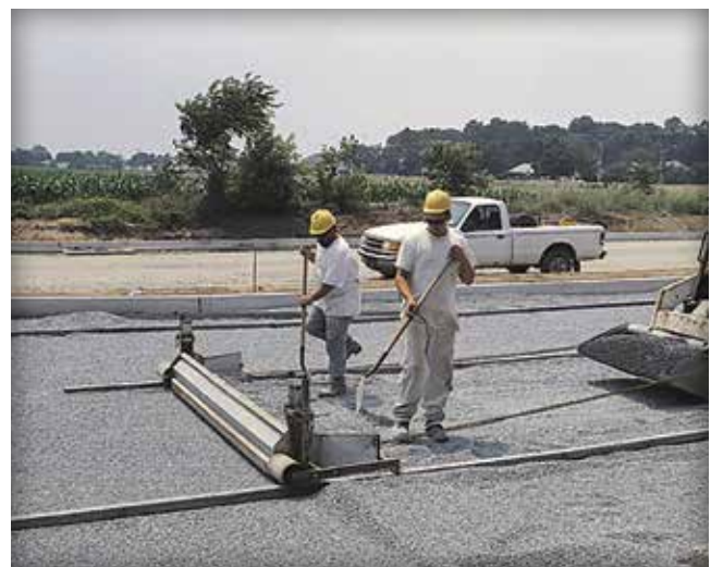
Figure 26. A screed beam pulled by equipment can be more efficient and productive.
